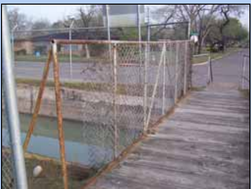
The drainage canal at South Park acts as a barrier but also presents as a safety concern due to poor fence maintenance along the bridge that crosses the canal.
