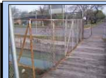
Fencing at one of the entrance points to South Park presents a safety concern.
